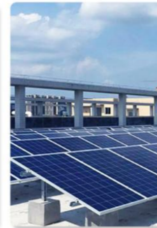
SOLAR ENERGY STORAGE
